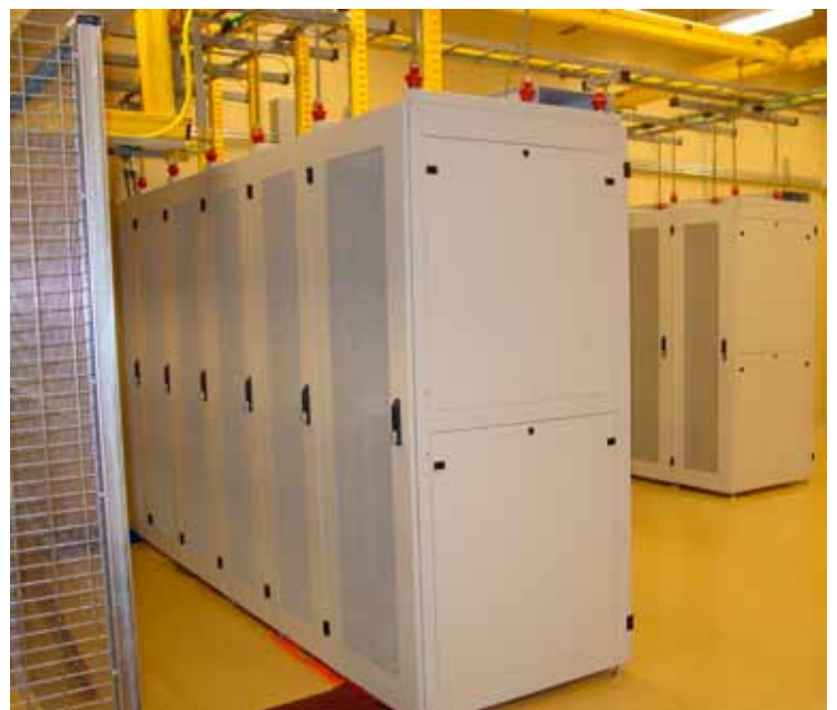
Co-location space includes equipment racks that can be leased in increments
